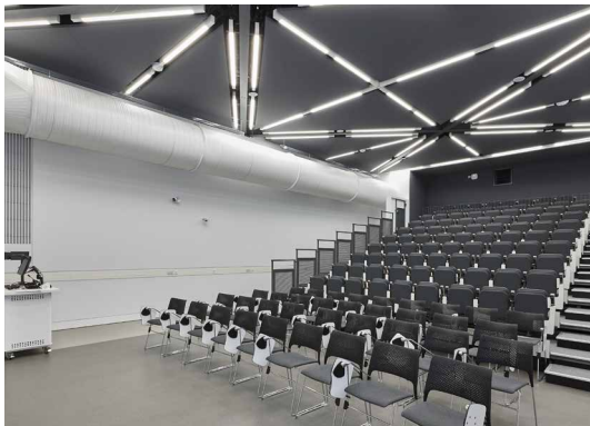
AGRG Winchester School of Art UNITED KINGDOM Photographer: Anthony Greenwood Photography Design: Absolute - Products Uses Installation: ACOUSTIC GRG
