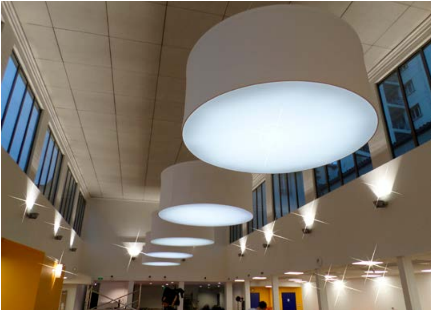
Shopping mall - XXL light fixtures in aluminum structure - Backlit coverings - France - Application : SPIDER DESIGN
